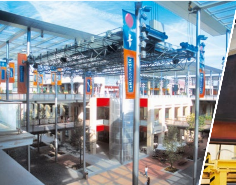
Synchronised DH hoist units lift and lower a roof segment in a shopping centre
