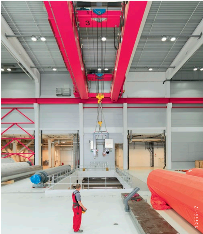
Load handling at two operating levels: Demag crane in stock preparation
