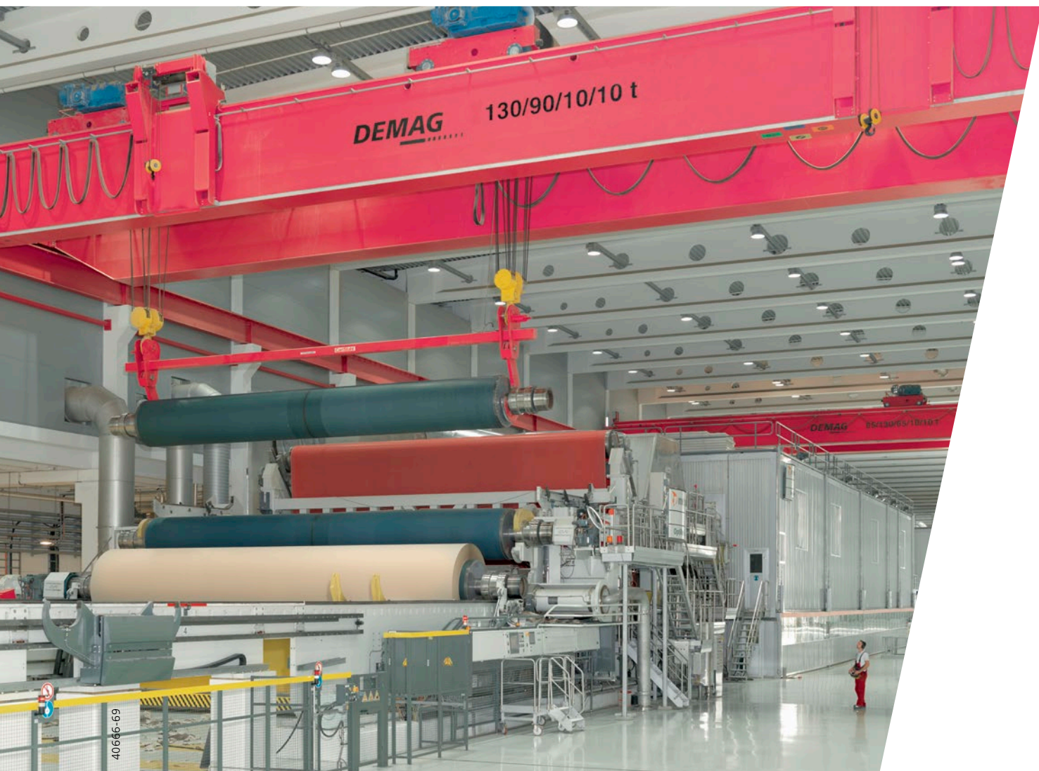
PM2: Demag cranes in production and maintenance
