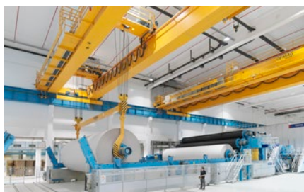
Process crane at the dry end of PM 7
